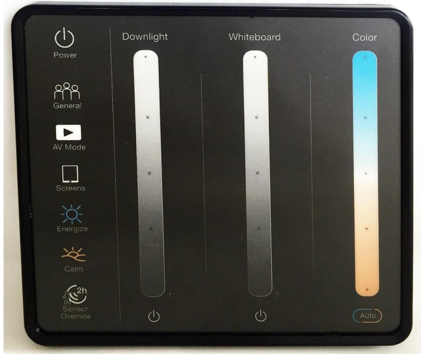
Figure 3. The Finelite LED lighting system control interface.
