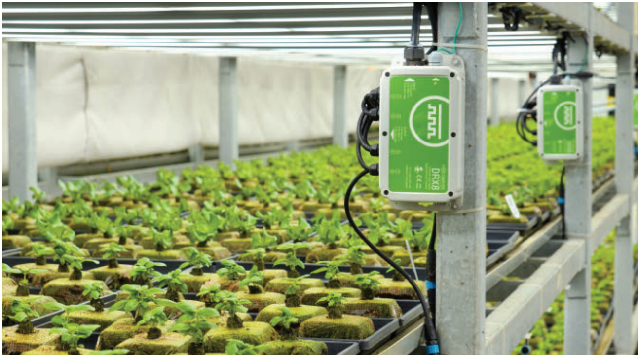
Receivers like these in the Hardee Fresh facility safely distribute the DC power to LED fixtures and other hardware in the humid growing environment. VoltServer
