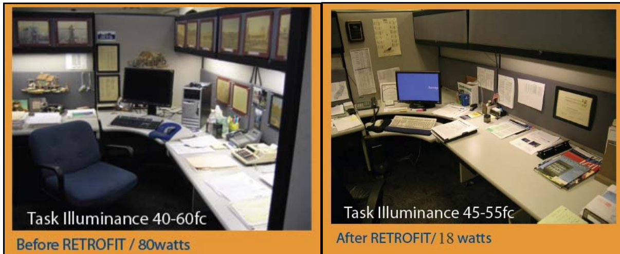
Figure 19. Example cubicle at the DMV office in Sacramento with undercabinet fluorescent task lighting system before retrofit (left) and PLS after retrofit (right) which yielded an 82% energy savings from lower wattage lighting combined with occupancy sensing controls.
