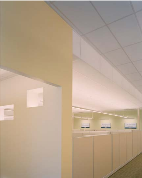
Figure 5. Example of low ambient design using 1 lamp high lumen T8 luminaires spaced 12' on center at an overall lighting power density of 0.5 w/sf.
