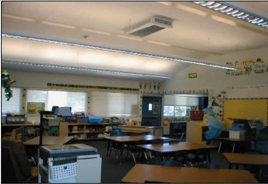
Country Club Elementary Control Room
